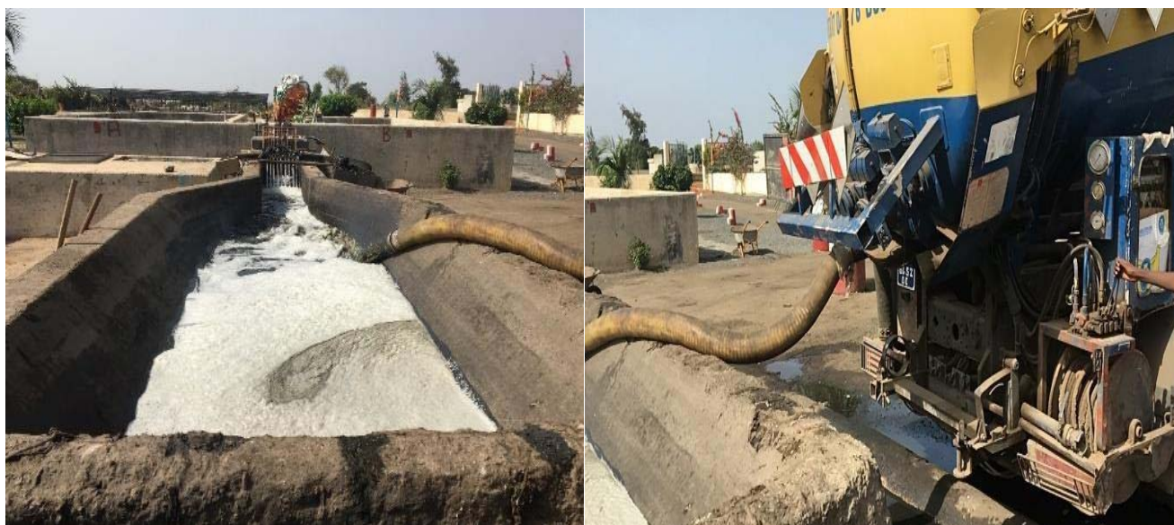
Fig.3: Raw sewage collection and screening
