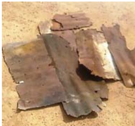
Plate 2. Used metal roofing sheets
